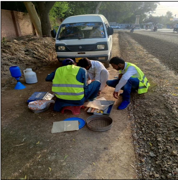
Picture 63: Field Density Testing on Aggregate Base 1st layer at Iqbal Road
