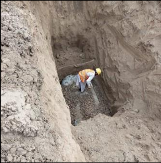
Picture 12: Construction of Manhole and Laying of Pipes at L2.5 42" Dia in Progress
